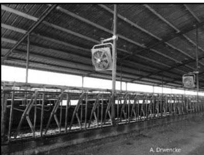
Fig. 2: Fans placed so that they cool cows at the bunk; moving air over wet animals removes more heat than when they are dry and means we need less soaking overall.
